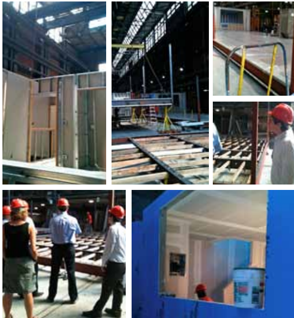
Recent tour of a modular construction factory based in Brooklyn with Cypress Hills Local Development Corporation.
